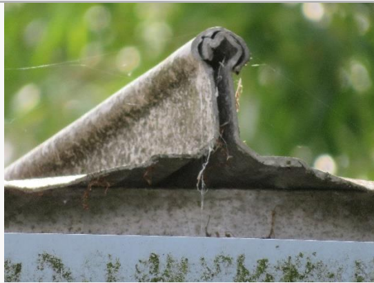
Photo 3: Corrugated sheeting: the pleats or folds form accessible voids
