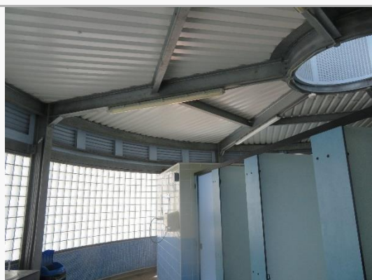
Photo 1: Female changing rooms, no roof void.
