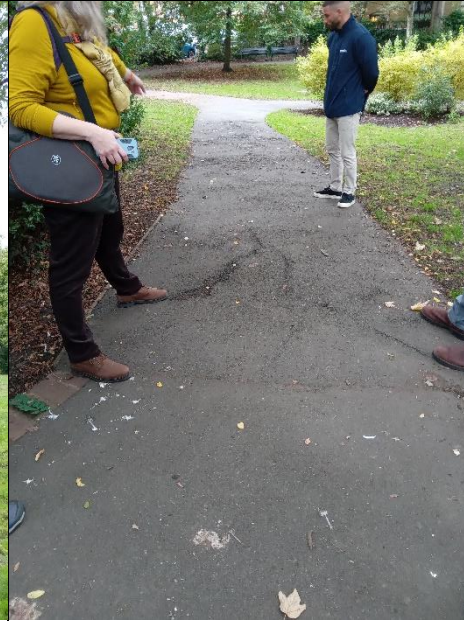
Tarmac path in need of repair
