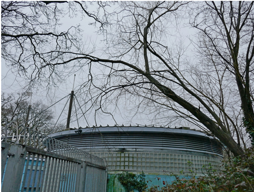
1) Tree 3 showing acute lean and damaged edge of the roof
