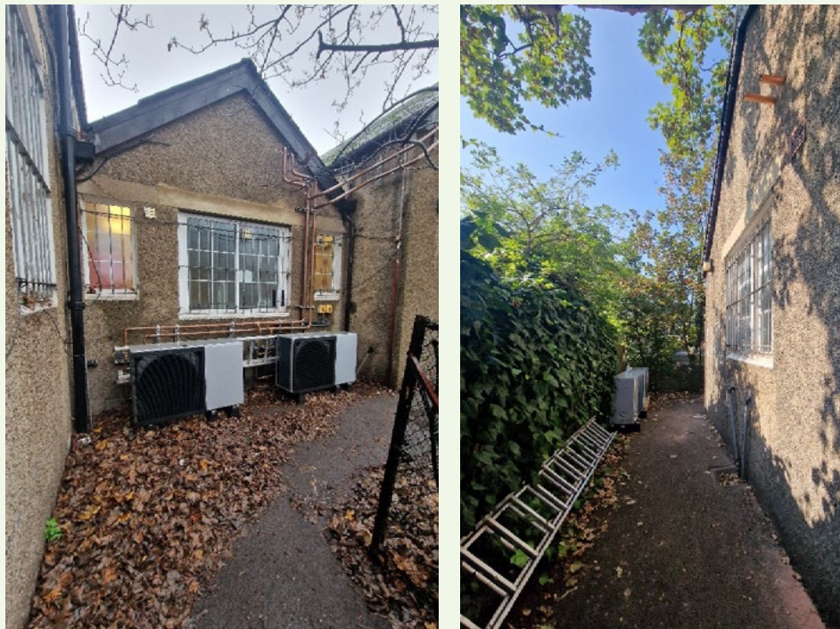
Air source heat pump at the Tooting Hub
