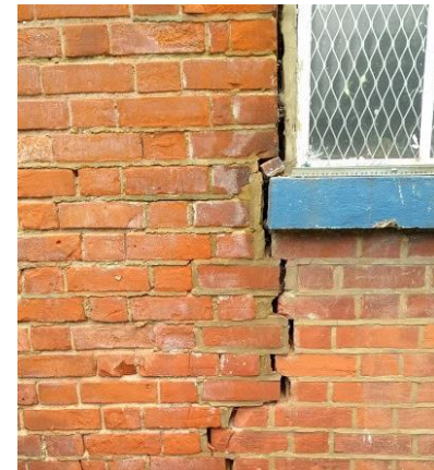
Typical wall cracking
