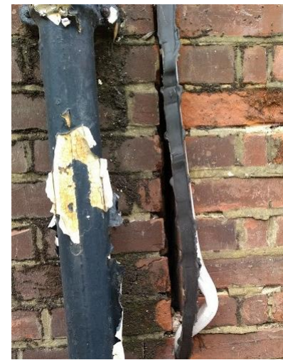
Cracking between rooms
