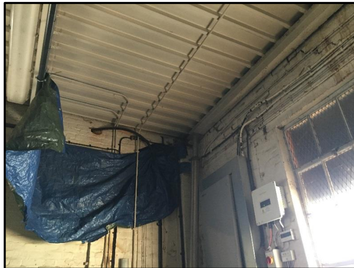
Photo 4.7: Pump house, internal, facing south west.
