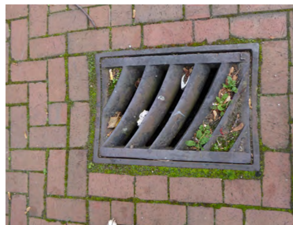
Route 1 - grill slots are too wide in gratings - can catch and break white guidance canes
