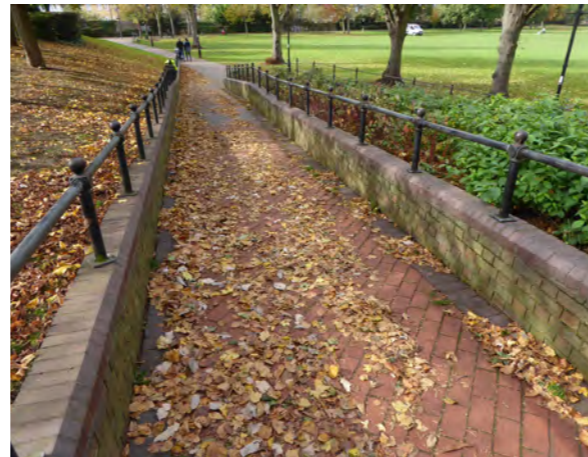
Route 1 - gradients are non-compliant and poorly managed for leaf clearance.
