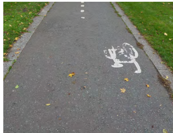
Route 1 - poor segregation and wearing off
