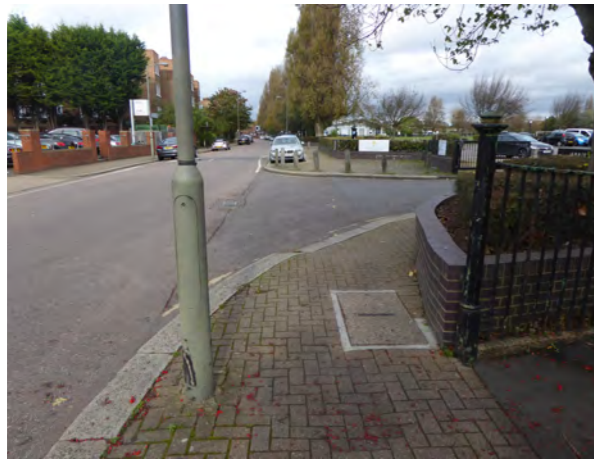
E6 entrance - lack of dropped kerbs / tactile paving
