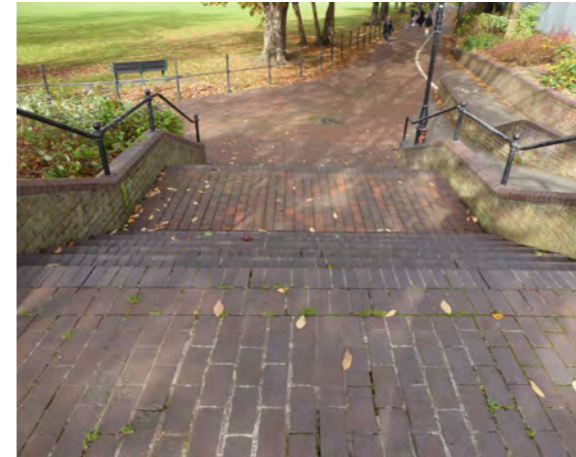
Route 1 - step nosings not highlighted, no tactile floor surfaces and central handrail required.
