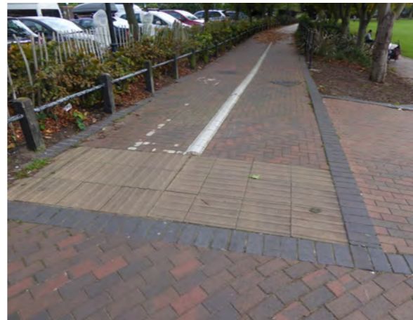
Route 1 - side on approach to cycle lanes from park - insufficient segregation
