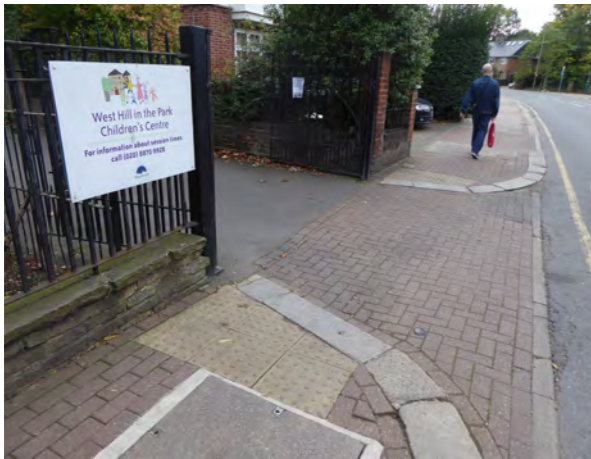
E14 entrance - uneven paving slabs
