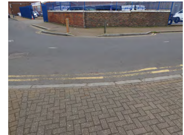
E4 entrance - inconsistent dropped kerbs and no tactile paving
