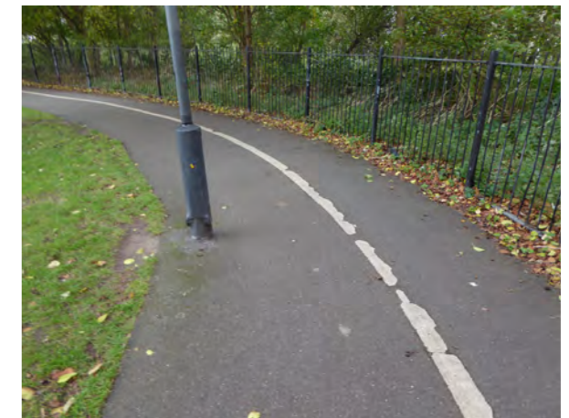
Route 1 - lampposts restrict widths en-route on pedestrian side
