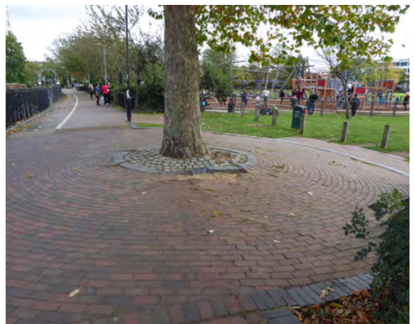
Route 3 - trip hazards
