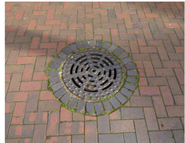
Route 2- some drainage grills may require resetting
