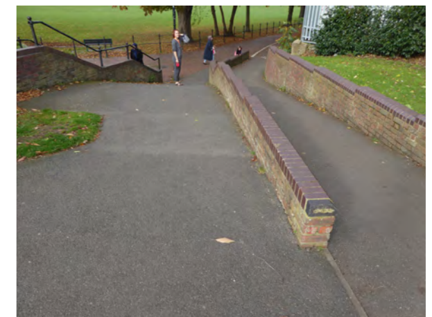
Route 1 - low level wall a trip hazard for blind and partially sighted people
