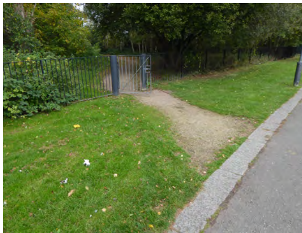
Route 6 - poor surfaces and raised kerb edge
