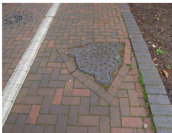
Route 1 - trip hazard from raised manhole covers
