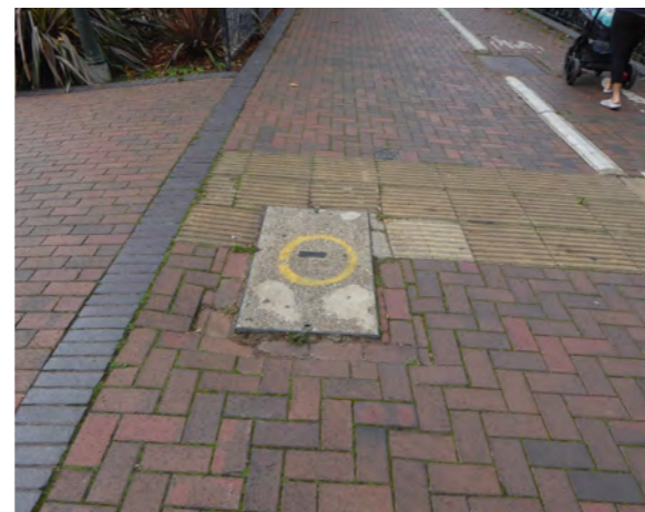
Route 3 - trip hazards
