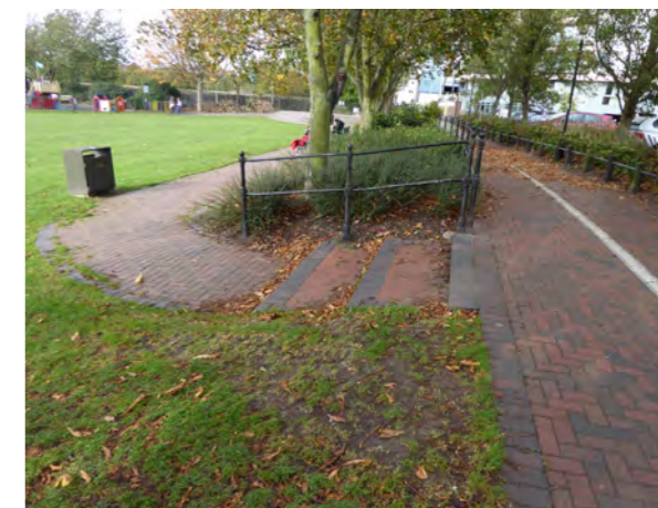
Route 1 - no tactile warnings on steps and poor step nosing definition
