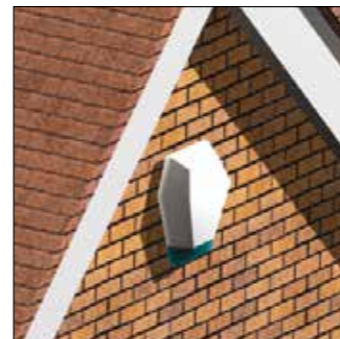
Front active alarm bell box
