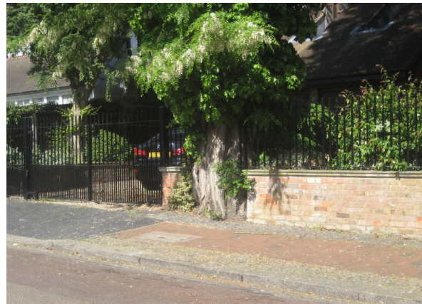
Figure 22 : Modern railings that are out of character with the conservation area
