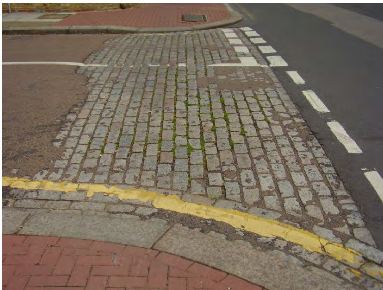
Figure 86 : Original granite setts surviving underneath the tarmac as they do in many places
