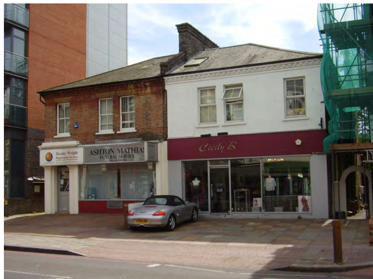
Figure 121 : Wide open featureless paving with car parking spoils the setting of these shops
