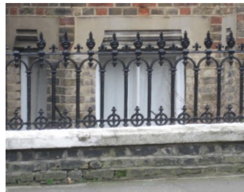
Type 2: Part of a complete run of original railings between 74-86 Grayshott Road
