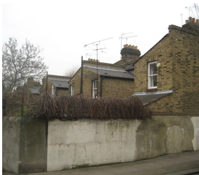
Figure 14 Regular and often unspoilt rear elevations and roofscapes can clearly be seen in many parts of the conservation area.
