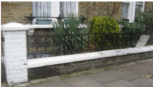
Figure 29 These railings have a modern design and are much thinner than the originals. Also the brick gate pillar should not be painted, but the bricks left bare, as is the case for all brickwork in the conservaiton area
