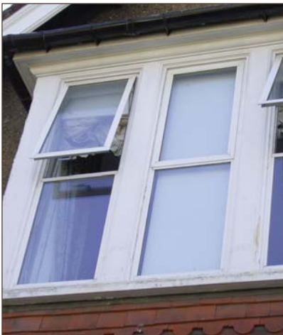
Replacement windows with unsuitable opening mechanism – should be sliding sash.
