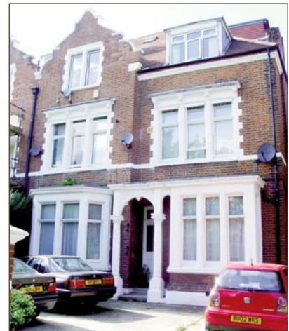
Four satellite dishes erected upon the front elevation detracts from the character of the house.
