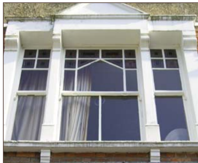
Timber tripartite sliding sash windows with intricate glazing members, decorative mullions and classical pediment lintel.
