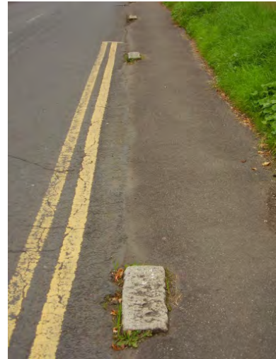
Figure 53 Granite kerb stones with unfortunate double yellow lines spoiling their appearance
