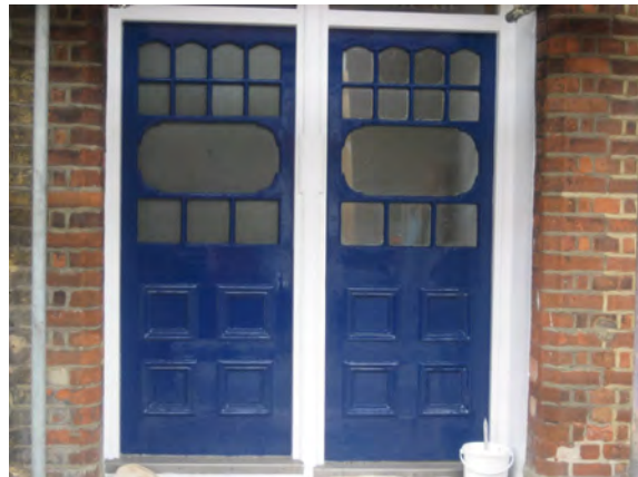
Figure 26 : A pair of original doors to the flats in Queenstown Road seen on the left
