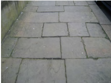
Figure 32 : Original York stone paving seen in St Philip Square and Broughton Street
