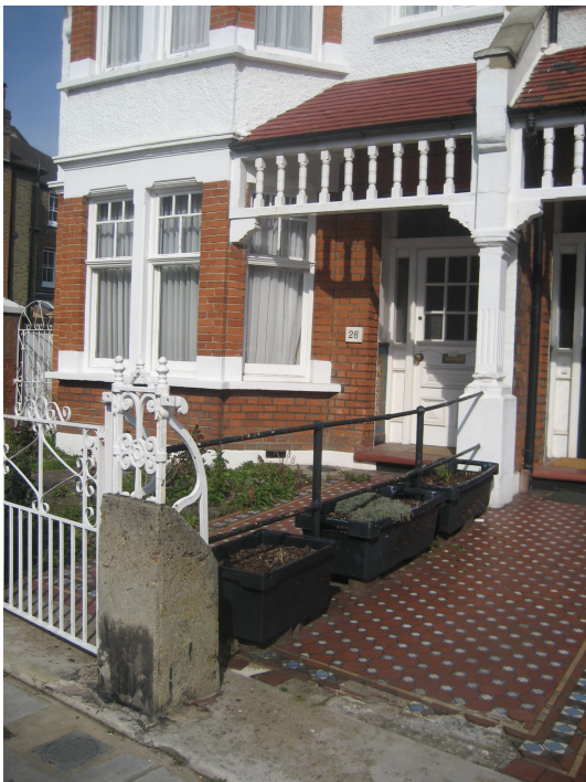
Figure 8 A rare survival of original cast ironwork. The simple rail dividing the two paths is probably also original
