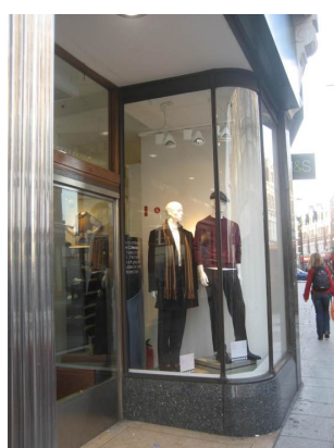
Figure 16 : The original bronze shop window at Marks and Spencer. A chrome column is just visible to the left
