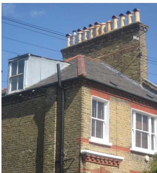
Figure 75 : A full set of chimney pots in Redgrave Road. The slate roof is an original finish and the dormer is suitably small and traditionally designed
