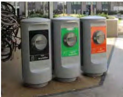
Figure 9.5: pneumatic waste collection system at Wembley
