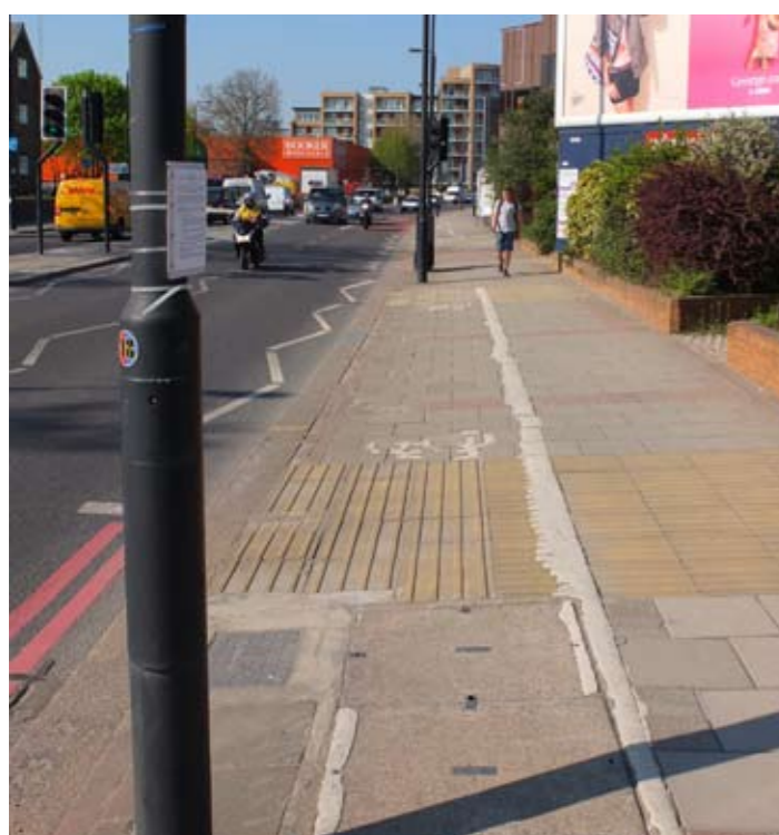
Unsafe, highly obstructed off-carriageway provision
