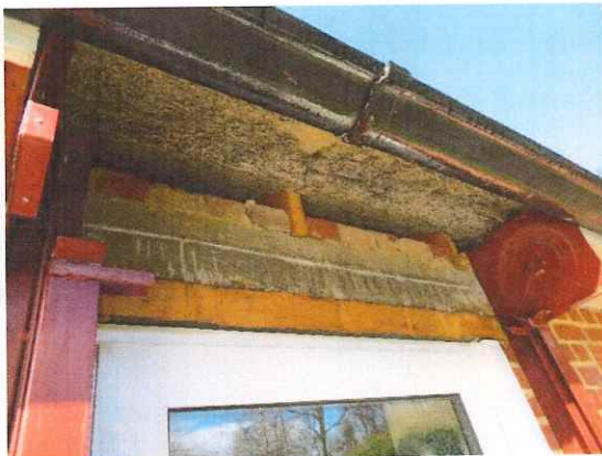
Photograph 3. Missing metal canopy with gap at eaves above door
