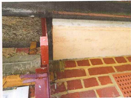
Photograph 4. Gap at soffit (area adjacent to photo 3)
