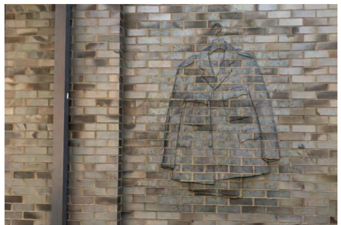
Fig. 413: Careful use of brick detailing within the semi-public space at the base of this development (Peabody Estate, St John's Hill) near Clapham Junction provides a human scale to the building.
